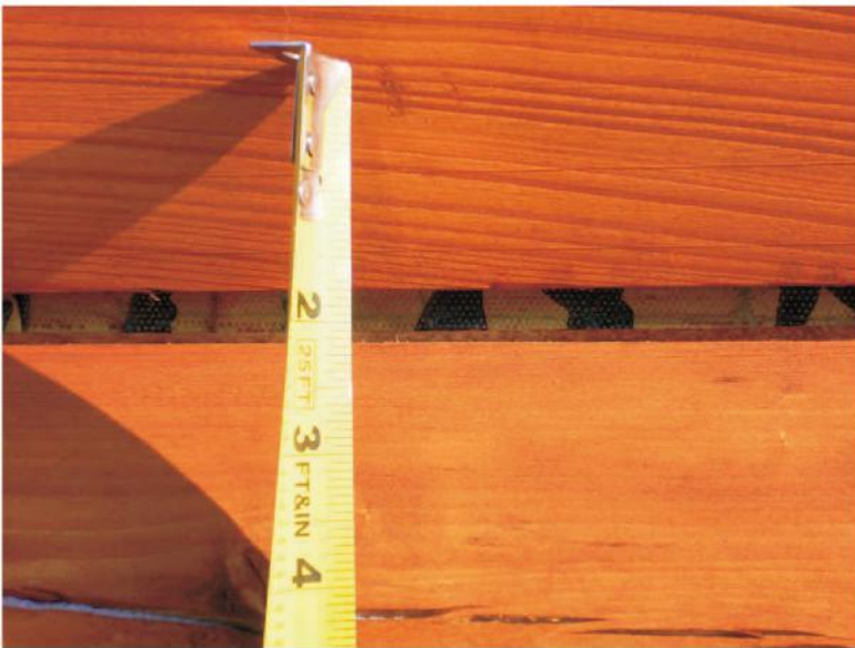
Gap created between siding courses.
