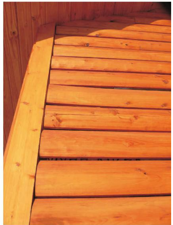
Twisted and warped siding.
