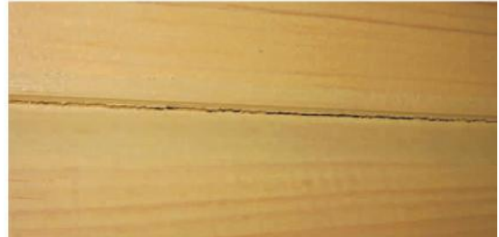
Split along siding seam.
