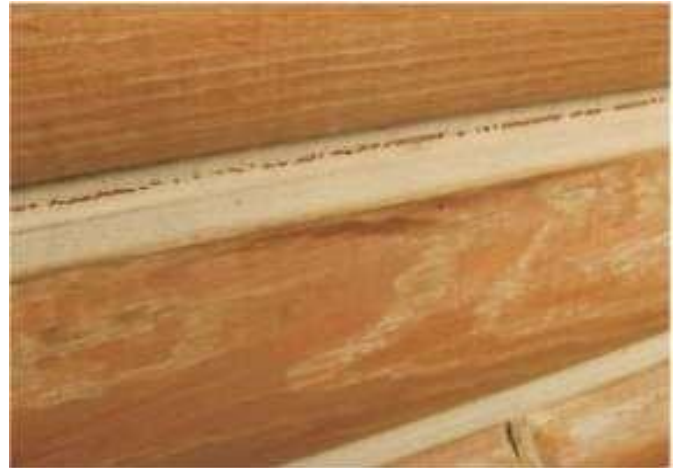
Chinking Applied Too Thin. Cut Out and Replace.
