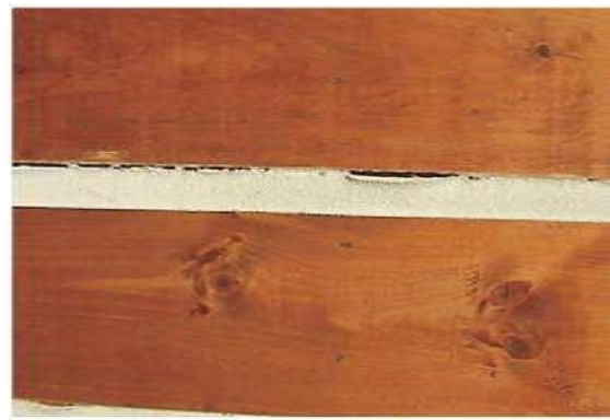
Tear That's Too Long to Repair.
