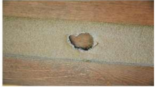
Blister Formed When Thin Layer Was Applied Over Improper Backing, In This Case Bare Wood
