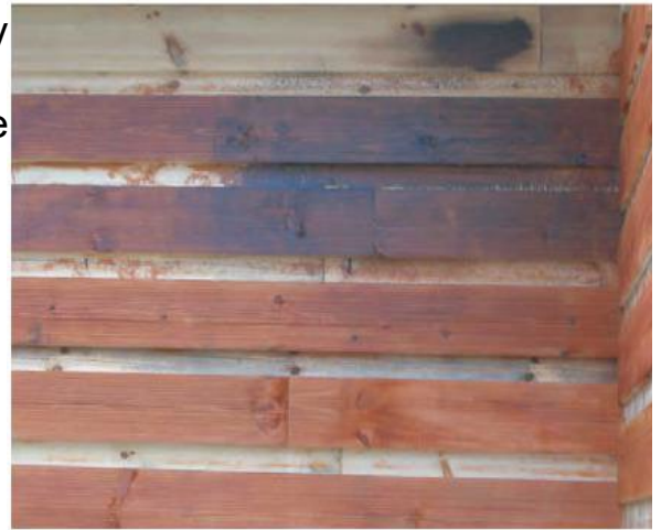
Inadequately mixed stain applied to wall.
