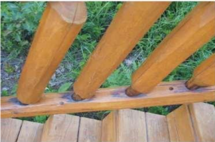
Exterior Water Stains Under the Finish
