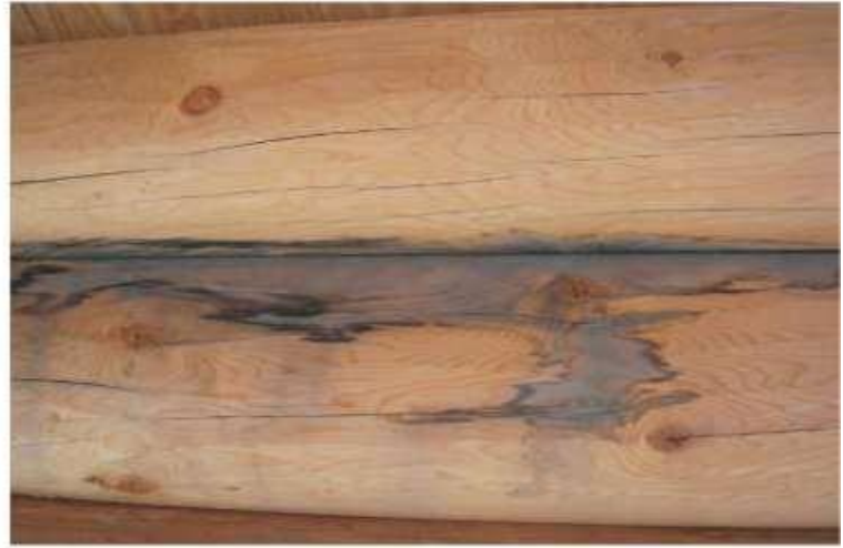
Interior Water Stains on Bare Wood
