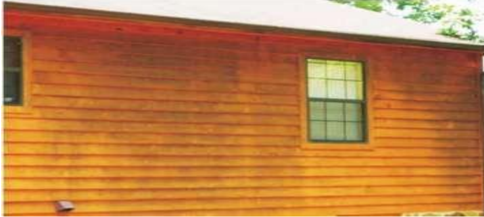
Iron tannate stains that appeared several months after the finish was applied. You can easily see where the bleach and water cleaning solution was inadequately rinsed.
