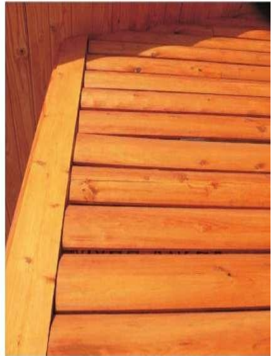
Twisted and warped siding.
