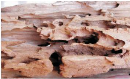
Carpenter Ant Damage
