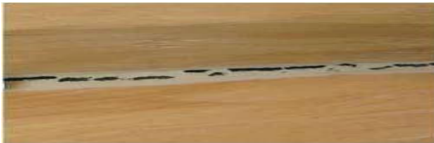
Sealant applied without a backing material to a joint between unseasoned logs
